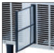
Proximity condenser air filter
