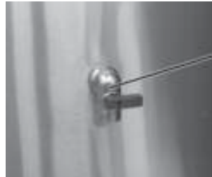
Control valve of steam generator
